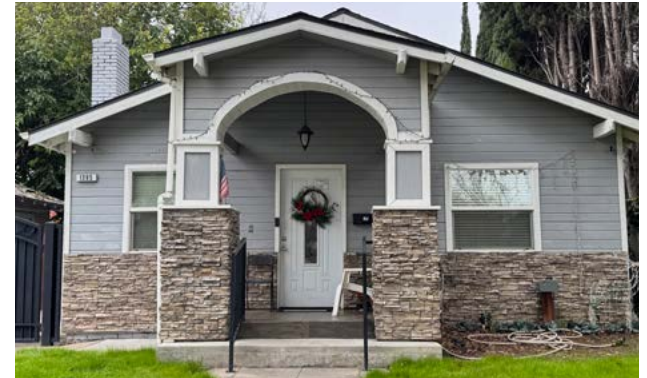
Stacked Stone. Stacked stone is not allowed, as it is a veneer with no possibility of structural purpose.
